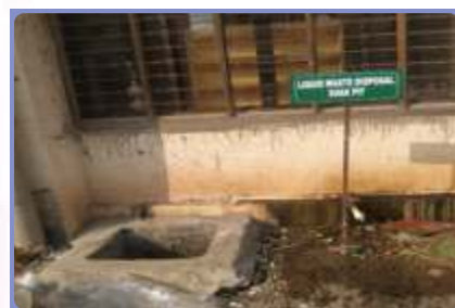
Liquid Waste Management Pit
