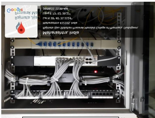
Cable network of internet in office
