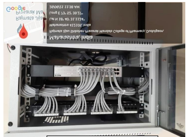
Cable network of internet in Computer Lab
