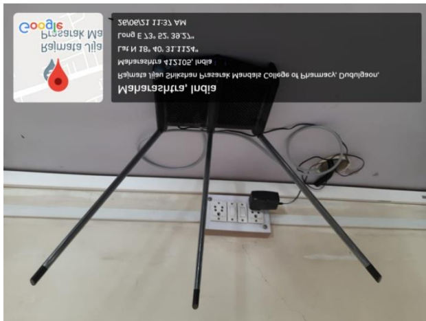
Connection of cable to router in computer lab
