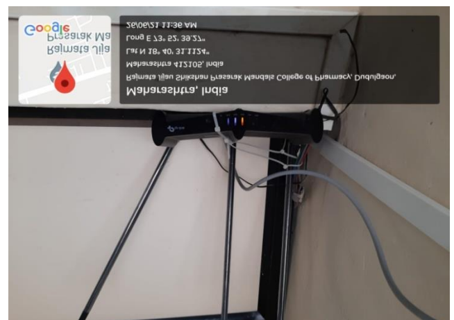
Connection of cable to router in office
