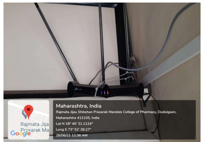
Connection of cable to router in office
