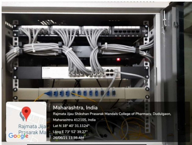
Cable network of internet in office
